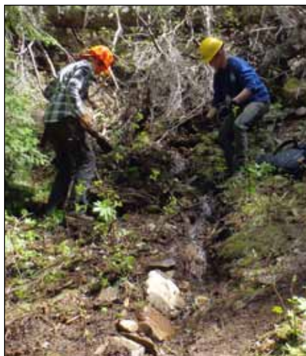
Marla Groot Nibbelink and Emily Cleveland divert a stream out of Trail #57 during Crew Leader College.
